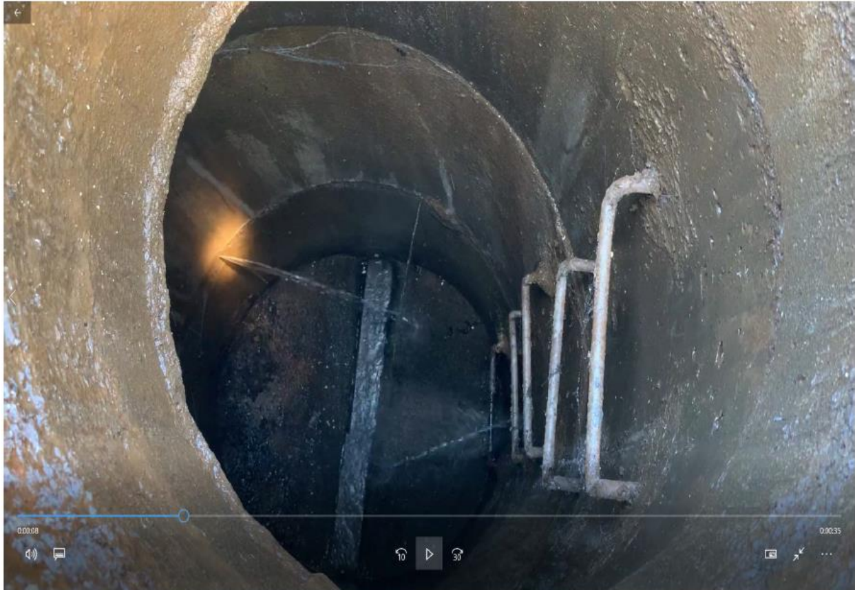
Figure 4-52 HVLCSD – Snapshot through Manhole Cover - Infiltration into Sewer Lines
