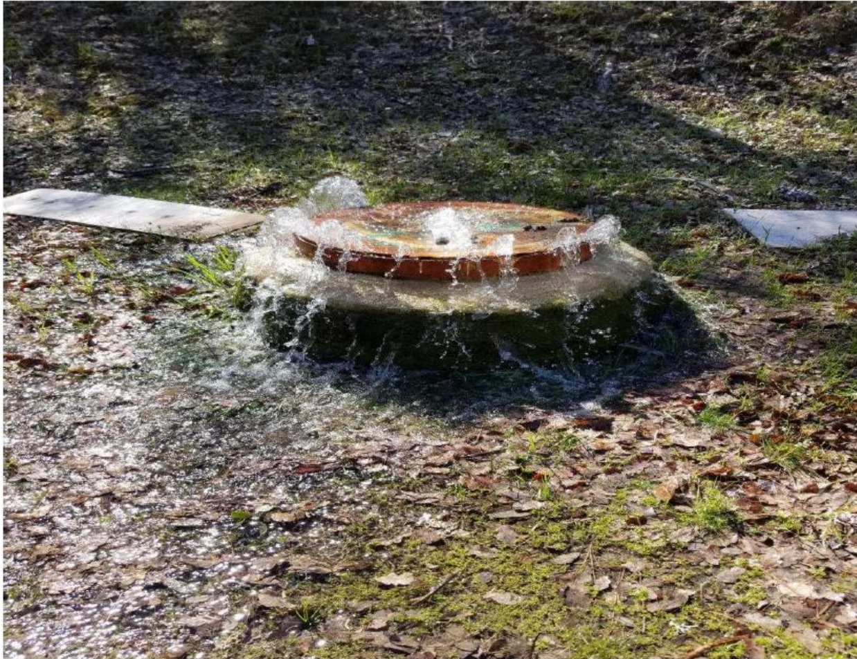
Figure 4-54 HVLCSD – Sewer System Overflow
