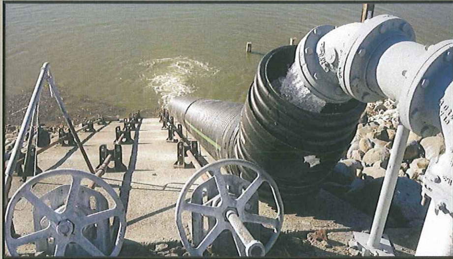
Reclamation pond release gates, repair was performed on the concrete base while pond is at a record low.
