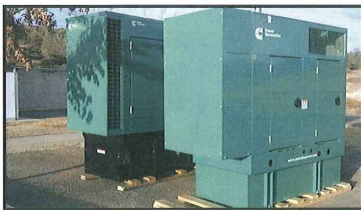
Generators for Lift Stations 1 and 4.
