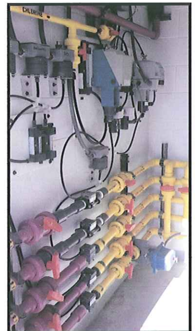
Installed chlorine control valves for the filters.
