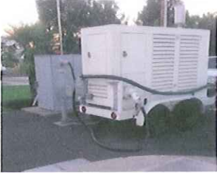
Generator in use at lift station 1 during power outage on Aug. 12th.
