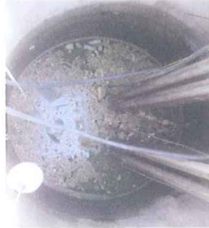
Lift station grease.
