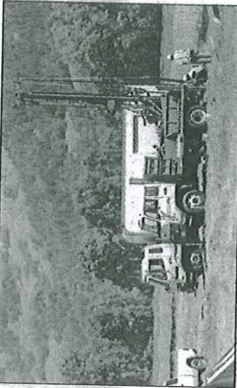
A CalTrans drilling rig working on the Willits bypass project in 2013. More than 100 boreholes were drilled in Little Lake Valley for this project.
