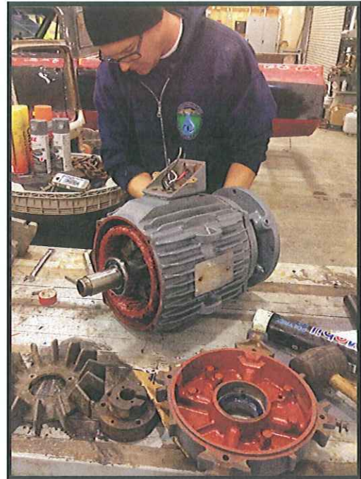
Barry working on motor from pump 400.
