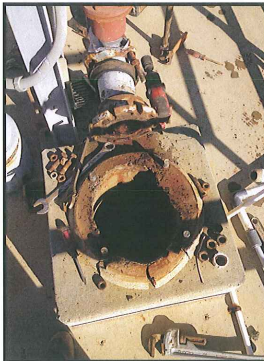
Well head after pump was pulled
