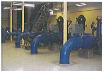
Photo: American Water High service pump station
