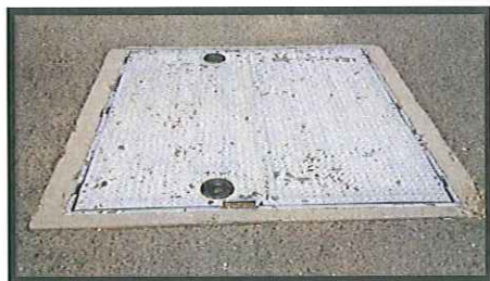
Lift Station 5 vault door
