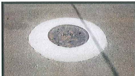
Manhole that was buried.
