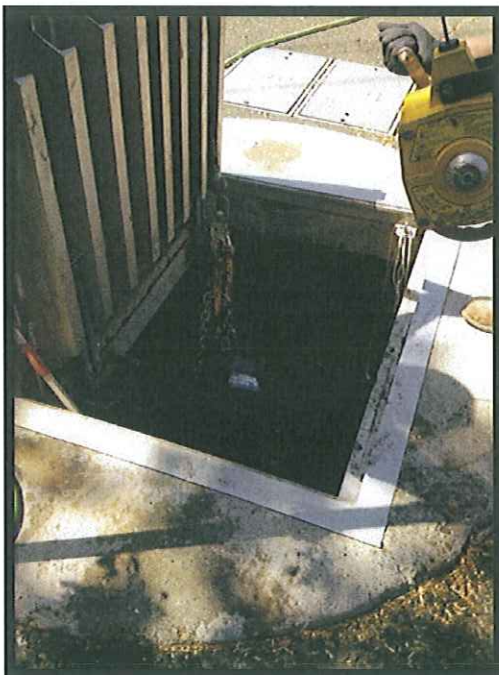
Lift station 3 pump #2 tripped again and was pulled to clean and fix it. Crane was down so we used the tri pod to pull the pump.
